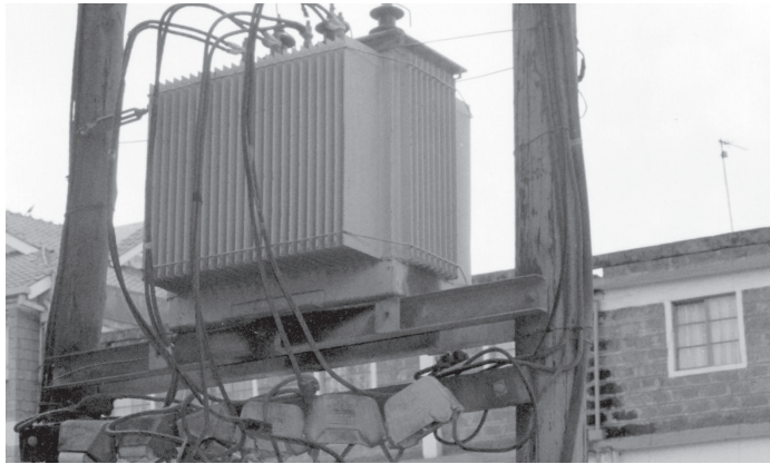
(c) A commercial step-down transformer
