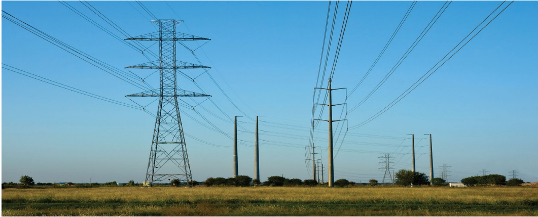
Fig. 8.15: Pylons and electricity transmission cables
